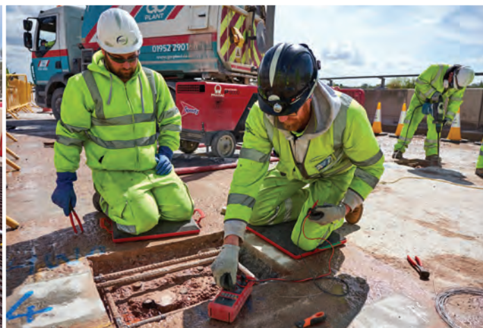
CRL's cathodic protection supervisor training an operative to carry out the continuity testing.
